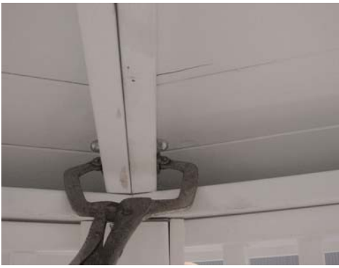
43. Use vice grip clamp to pull sections together and install bolts in rafters
