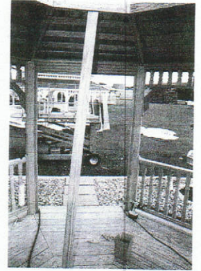
#26 - Using a prop cut to a length slightly longer than the highest point of the roof section may make assembly of the roof easier.
