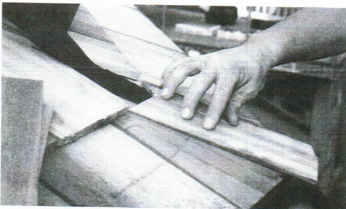
#40 - With the roof felt over the seam nail one half of the cap shingle on the bottom course.
