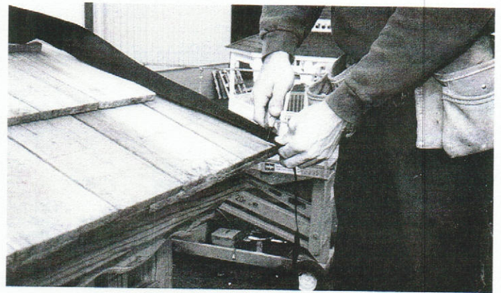
#39 - With roof sections in place and secure, cap the panel seams. Begin by measuring and cutting to length a piece of roof felt the length of each seam.
