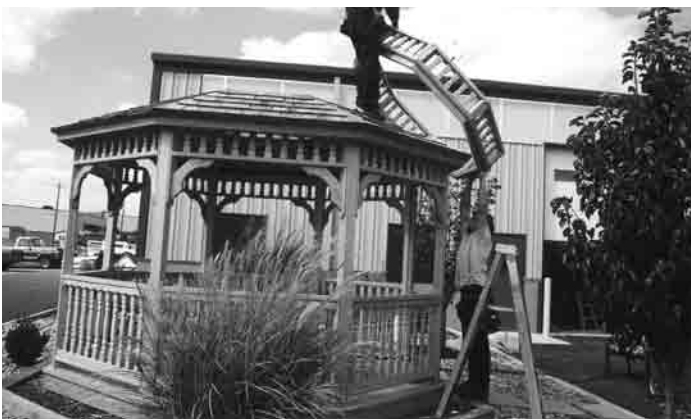
#P3 - With assistance, raise the railing section onto the roof and position as shown in hole.
