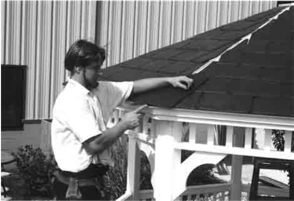
#33 - When roof is completed, cap seams of sections. Bend caps along center line with textured side out (in the case of shingles).
