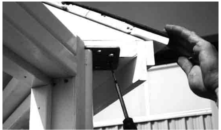
#28 - Drive (2) screws through roof bracket into roof 2x8 plate on both corners of section. Under normal weather conditions or without other additional pressure, roof section will stay in place until next section is positioned up to 14'. Bigger gazebos need center support.
