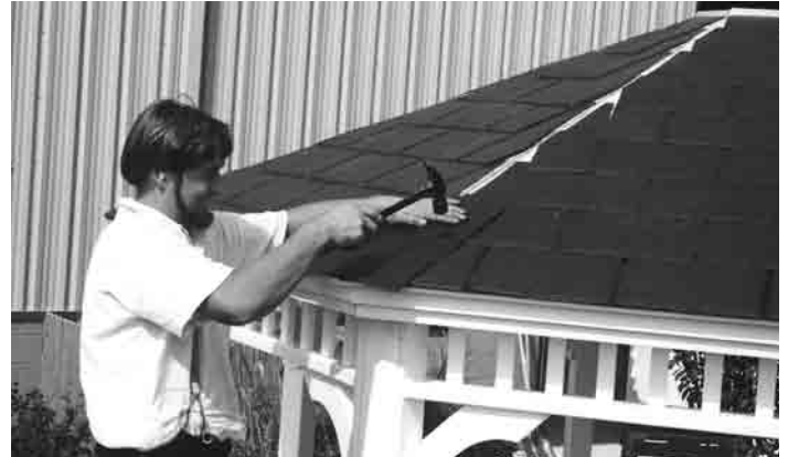
#34 - Align bottom of first shingle at bottom of roof and nail using upper hole on both sides.
