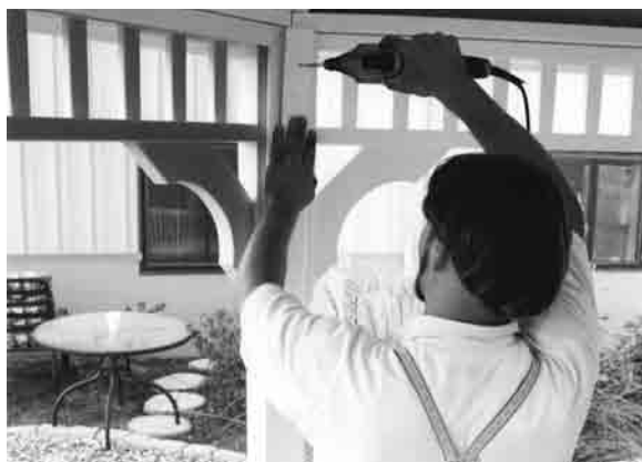
#39 - To install screens, center the panel in the opening opposite the door. Secure the screen panel in place using the “T” shaped trim shown in the next illustration (1).
