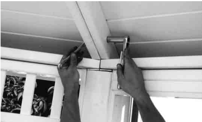
#31 - Secure with threaded rod and acorn nuts. (2-4 sets per rafter depending on size) Continue with one panel at a time until roof is complete.
