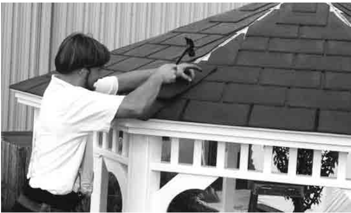
#35 - Second shingle is aligned with notch on shingle below and nailed in upper hole.
