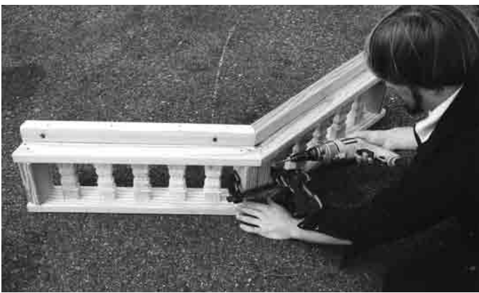
#P1 - Pagoda roof railing sections are screwed together on the ground, to form an octagon. (See picture 25)
