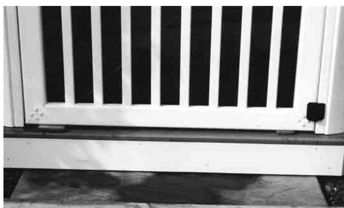
#41 - Reattach door hinges to jamb,
