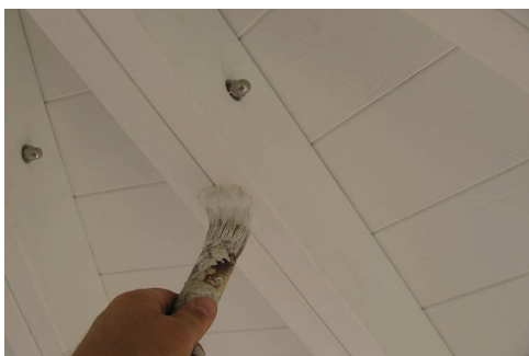
Go back over all painted section of the Gazebo and touch it up with the provided touch up paint.
