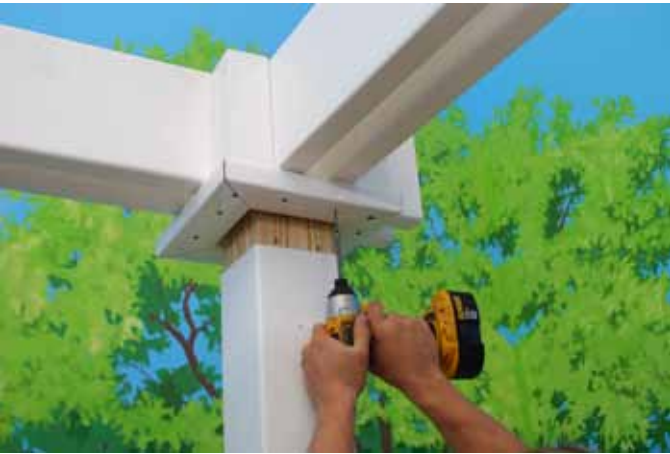
Fasten Square Trim to 2x8 Header Boards from bottom up using (2) 2.1/2" Brown Screws through pre-drilled holes.
