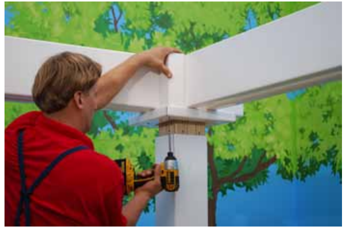
Fasten Square Trim to Inside Corner Trim from the bottom up using (1) 2.1/2" Brown Screw. Top side will get fastened later.
