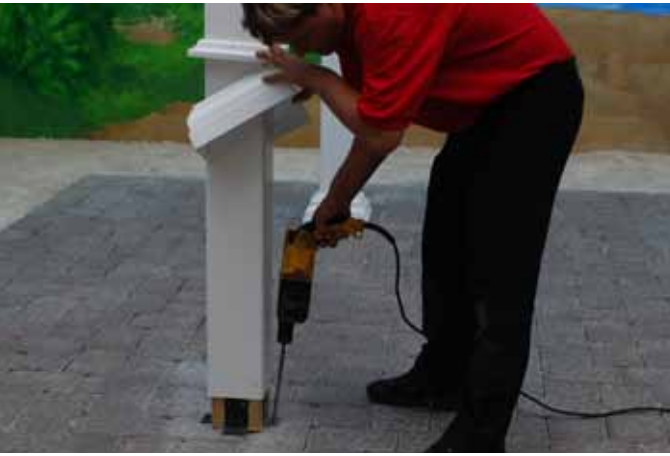
Anchor Post to Concrete Pier below. Pre-drill hole in concrete using a 1/2" cement drill bit.
