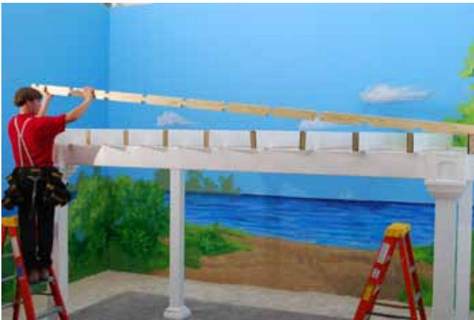
Use provided spacer board to place all 2x6 Rafter Joists into position.
