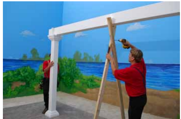
To keep the Header Assembly upright build an A-frame brace using your own 8' long 2x4's and fasten with (2) 2.1/2" screws.
